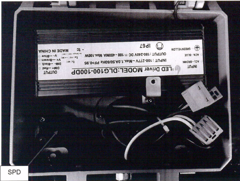
Picture 62.: Internal view for LED driver chamber
